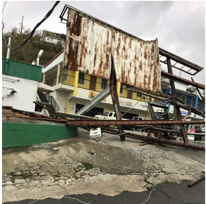
Wind damaged the Puma Gas Station in Smith Bay, St. Thomas after Hurricane Irma in 2017. (Source Photo by Diana Dias)
