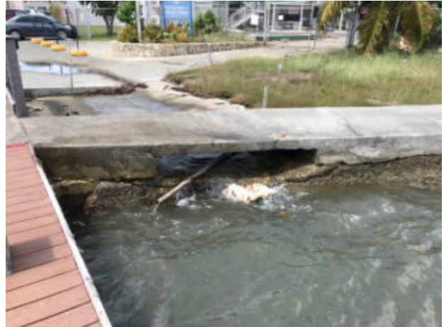
Drainage pipes near where the Christiansted boardwalk meets the seaplane terminal cannot drain properly with such high levels of seawater intrusion. (Source photo by Kelsey Nowakowski)
